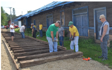
Laying a section of track from the Pittsburg, Shawmut, & Northern Railroad; the rails are original pieces that were laid where the train once ran through the current Hahn & Schaffner site
