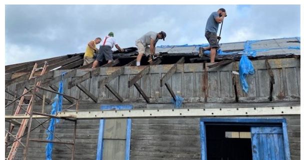
Removing the roof from the Pittsburg, Shawmut, & Northern Railroad depot; it was replaced with a metal roof (refer to page one for more information on both photos)
